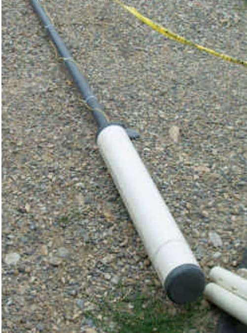
Photo 1 - Injection Well Screen and Riser
