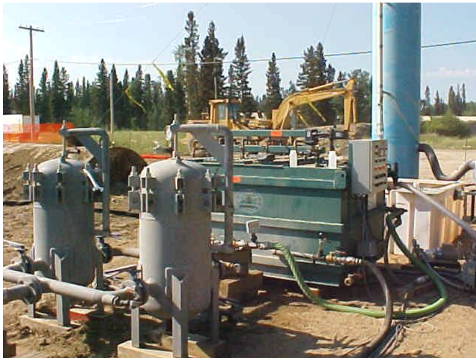
Photo 2: On-site Water Treatment System
